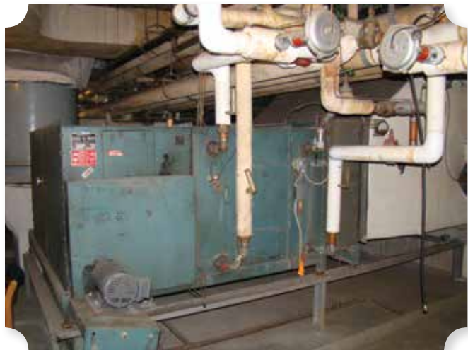
2015 photo of a mechanical system that has since been replaced.
